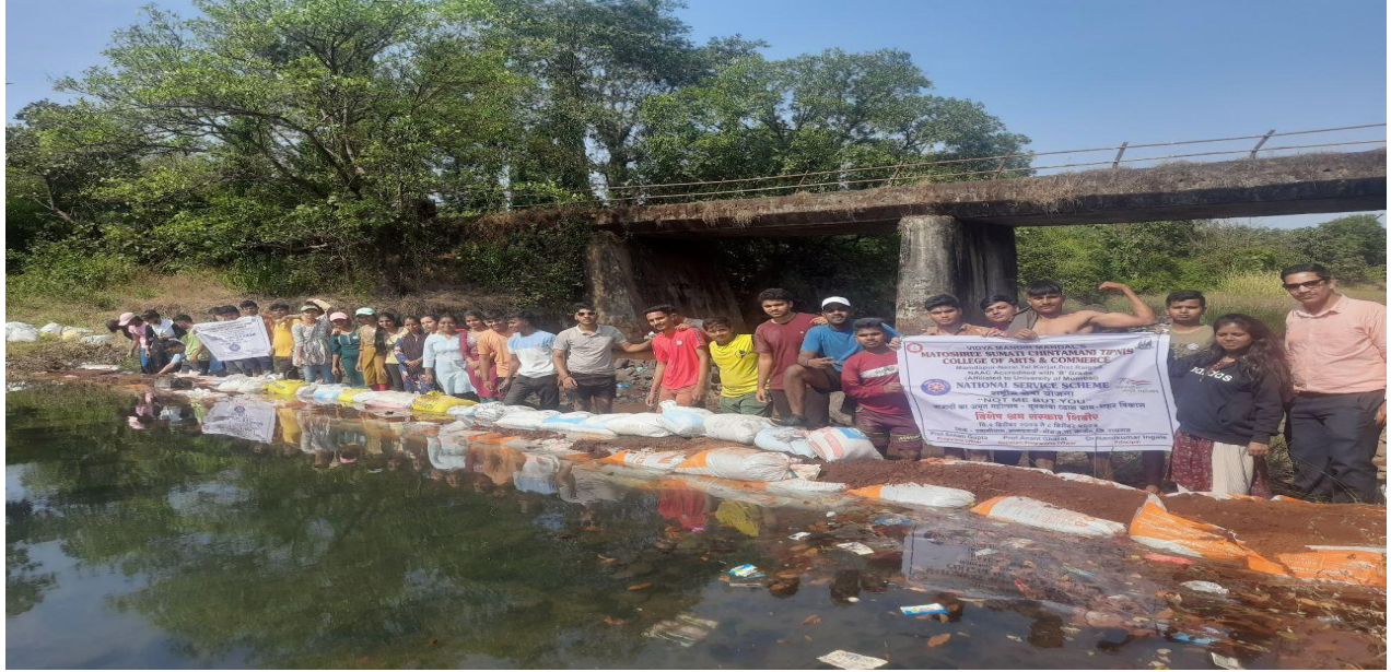
Construction of a bund on the river in Anandwadi village during the 7 Day Residential Camp
